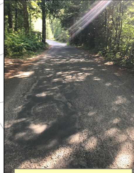
Peaceful Valley Drive pavement in poor condition at entrance patches, settlement, and cracking
