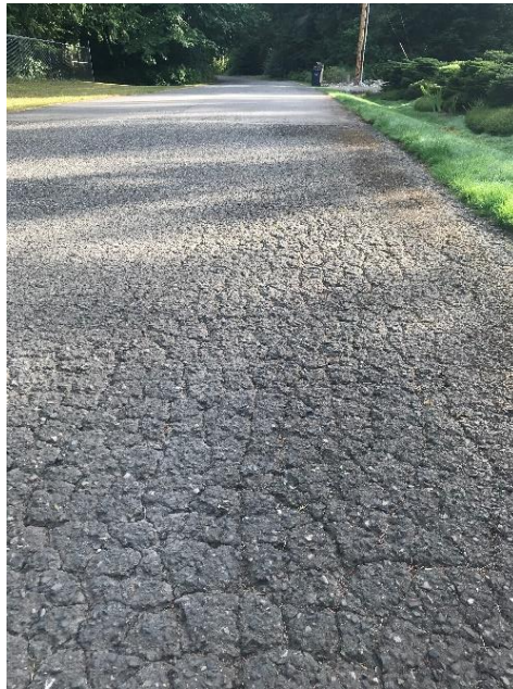
Sprague Valley Drive: Alligator Cracking
