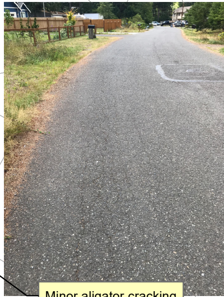
Minor alligator cracking
