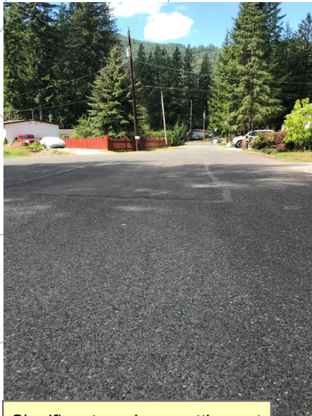
Significant roadway settlement
