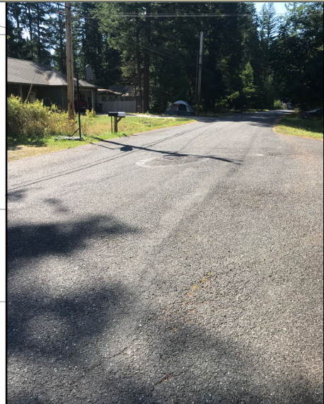
Significant roadway settlement around manhole
