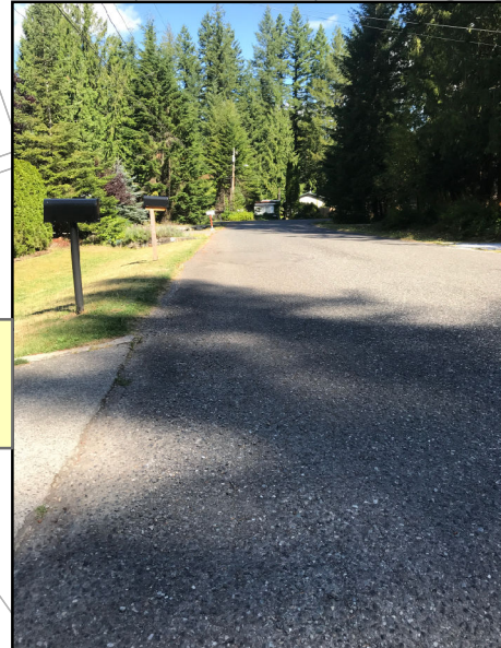
Significant roadway settlement
