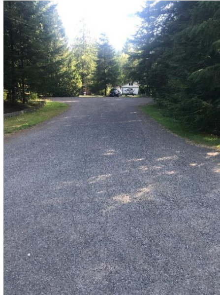
Happy Valley Court: Alligator Cracking
