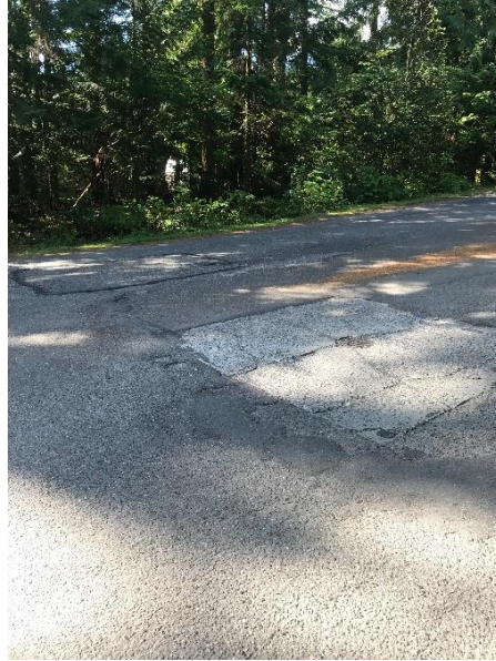
Peaceful Valley Drive: Poor Patch
